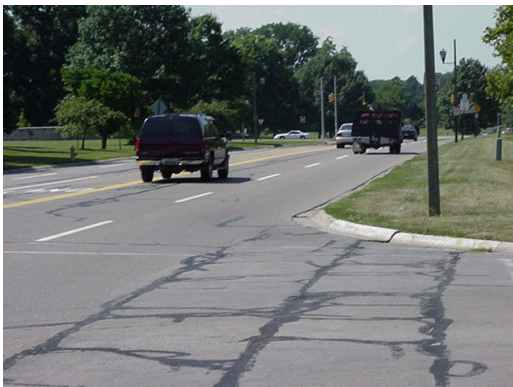
Kenny Road Looking North Near City Hall
