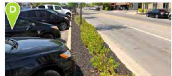
Missing sidewalk in front of Shops on Lane Avenue.
