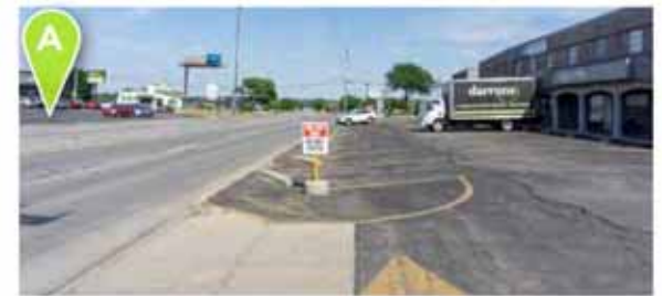
Missing sidewalk entering the corridor from West Campus.
