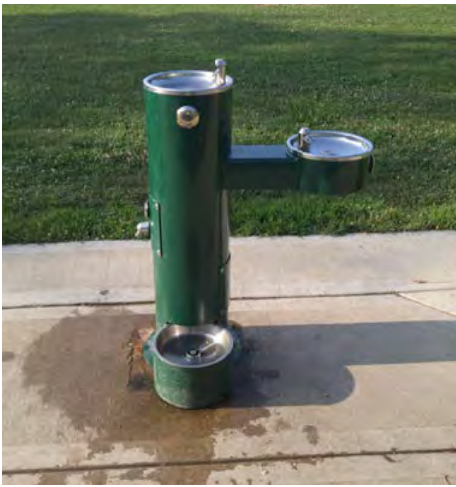
Drinking fountain at Tennis Building
