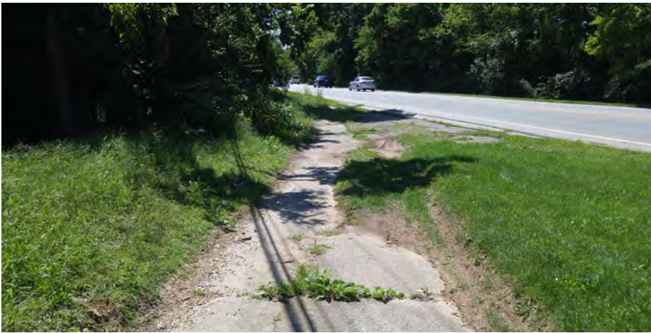
Broken up walkway ends into Riverside Drive
