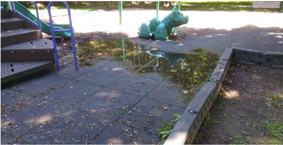
Playground drainage problem area
