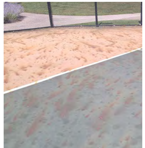
Discoloration on the tennis courts
